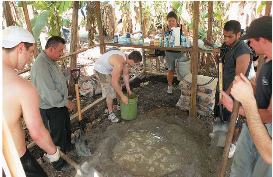
Northeastern University students help build a restaurant for Marina, a South African entrepreneur, as part of the Field Study Program.
